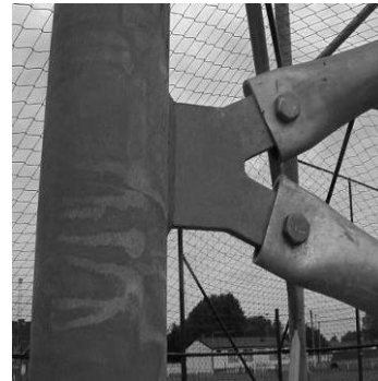
Figure 11: New joint between diagonal and leg, both circular tubes. KPN-Orange in Belgium
