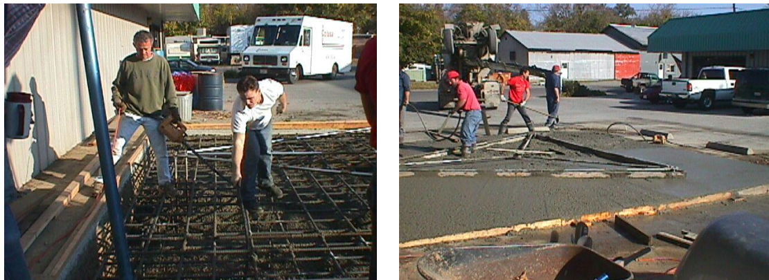
Image 8: a) Using a vibrator in the wet concrete to eliminate flaws such as honeycombs and air pockets. b) The central area should be flat with a brushed finish while the surrounding area is sloping (outwards) with a floating finish (completed only in the right corner).
